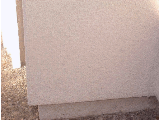
Visible mesh patterning through finish coat application indicates lack of proper amount of base coat at original application
