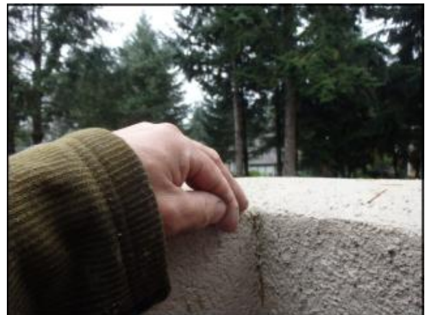
Cracking observed at deck wall and cap; deck wall and cap need elastomeric coating application
