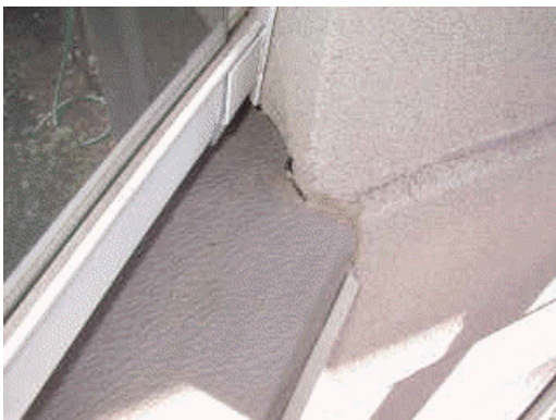
Deck termination needs end dam installed; elevated moisture readings obtained below; typical
