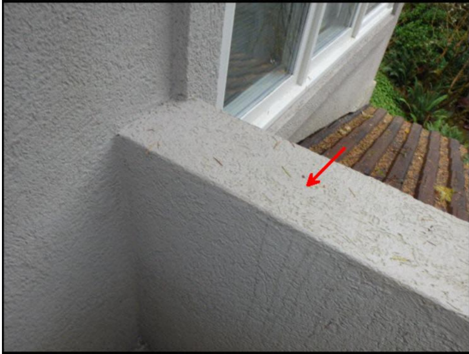
Non-sloped EIFS deck cap needs elastomeric coating application (D4-F3)
