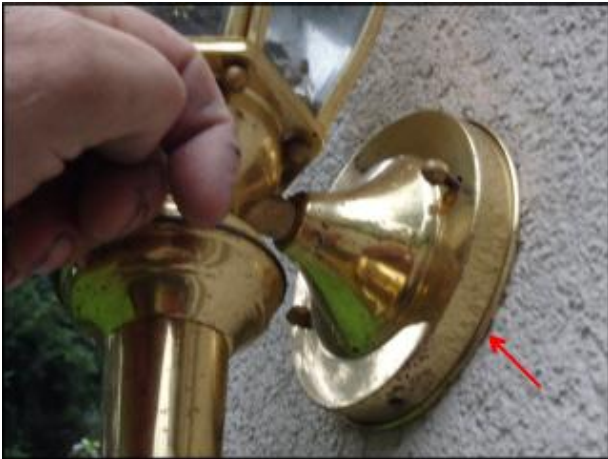
Light penetration needs to be sealed; typical
