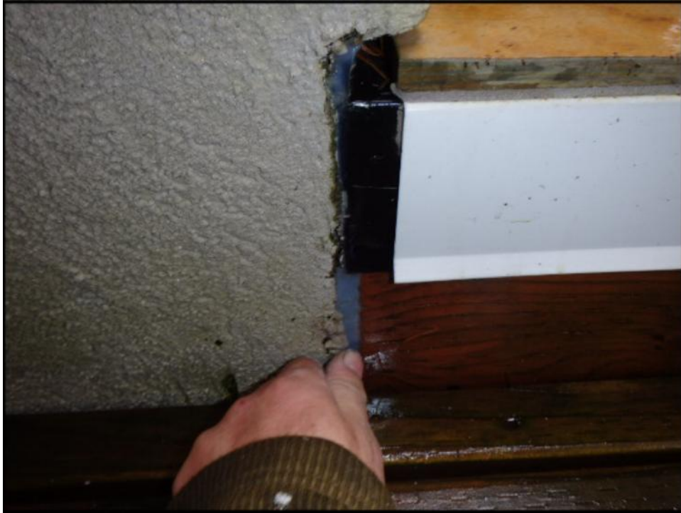
Sealant joint and end dam in good condition at deck termination (J8)
