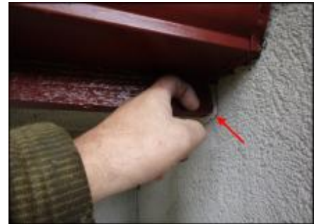
Sealant joint failure at fascia termination needs remediation (H3)
