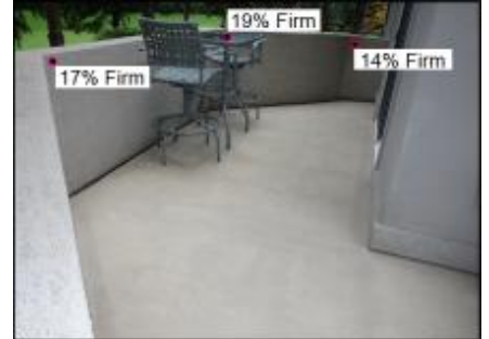
Moisture readings obtained at interior deck wall (F3-H3)
