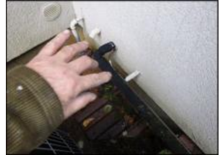
Penetrations need sealant joint application (A7)
