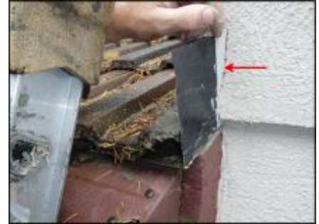
Roof step flashing needs sealant joint application (F4)
