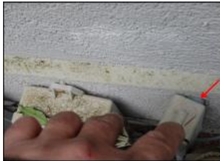
Penetration needs sealant joint application (C7)
