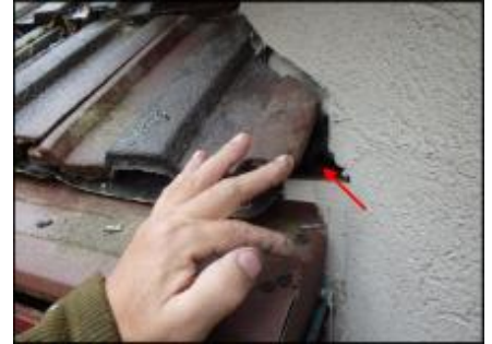
Roof termination needs flashing installed (B4)
