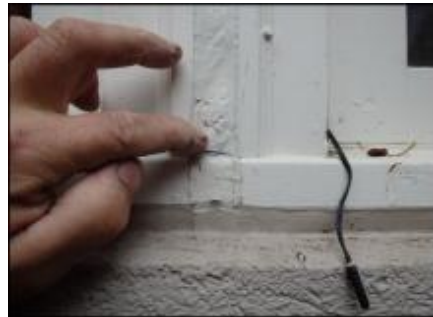
Area of thin sealant application at window mullion needs additional sealant application (A5)
