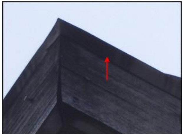
Flashing at chimney cap adequately extends over wood trim to protect against moisture intrusion
