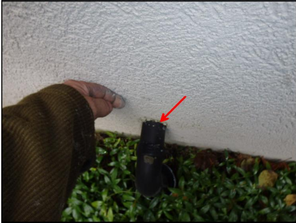
Penetration needs sealant joint application (H7)
