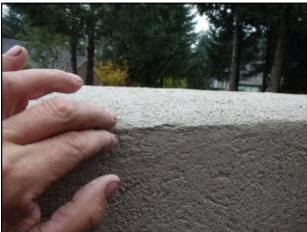
Cracking observed at deck wall and cap; deck wall and cap need elastomeric coating application
