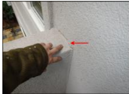
Crack at deck wall to dwelling wall needs sealant joint application (F3)
