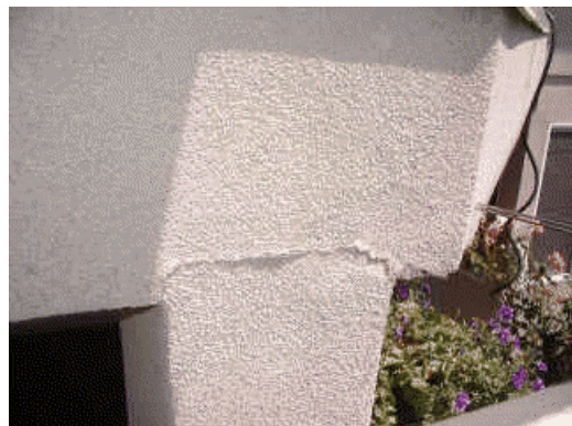
Area of compression cracking occurring needs remediation
