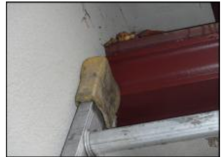
Leak at gutter end cap needs to be sealed (J1)
