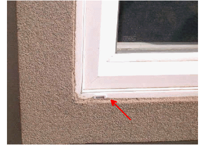
Window detail needs remediation to accommodate sealant joint and window weep hole; typical
