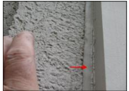
Sealant joint in good condition at garage door head and jambs; typical
