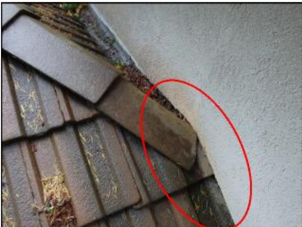
Dead valley needs to be cleared of debris to allow for drainage; recommend further evaluation to determine necessary remediation to allow for unobstructed water flow to gutter (I3-J3)
