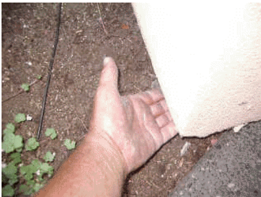
Exposed foam at base of system needs mesh and base coat application; typical
