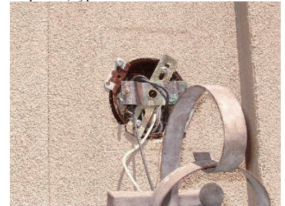
Light fixture needs sealant joint application
