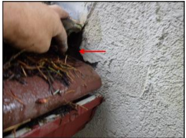
Exposed Sprock board at gutter termination needs base coat and mesh application (J3)
