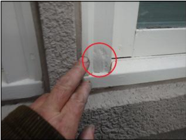
Area of wood rot at window construction needs remediation (I7)
