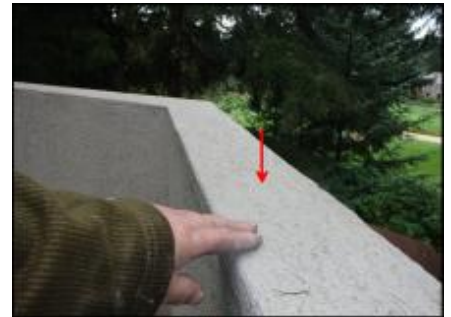
Cracking observed at non-sloped EIFS deck cap; deck cap needs elastomeric coating application (F3-I3)
