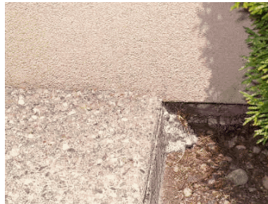
Concrete poured to EIFS not per manufacturer's specifications
