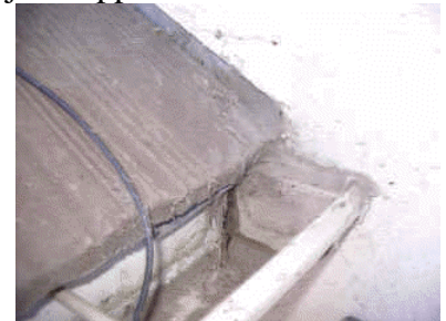
Roof termination needs kickout flashing installed
