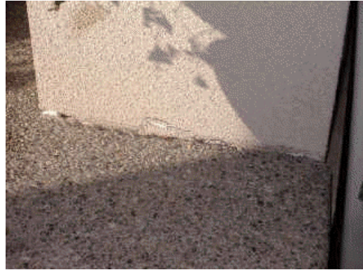
Settling and cracking occurring at concrete poured to EIFS; area needs flashing installed; typical
