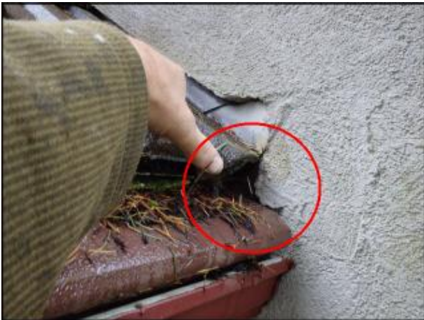
Roof termination needs one-piece (seamless) kickout flashing installed (J3)
