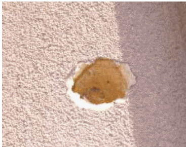
Bird damage needs remediation (B2)
