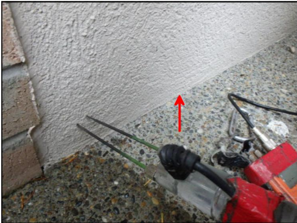
Low moisture readings obtained at concrete poured to base of system; detail can be remediated with sealant joint application; typical
