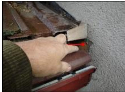
Exposed Sprock board at gutter termination needs base coat and mesh application (H3)
