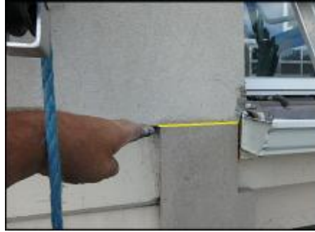
Area of compression damage needs expansion joint installation (H6)
