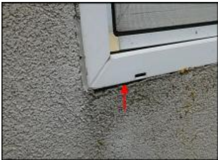
7/8" EIFS needs to be removed at window perimeter prior to base coat and mesh application to accommodate 3/4" silicone sealant joint application; typical
