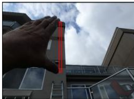
Approximate area of soft substrate needs to be removed and replaced (G1-H4)
