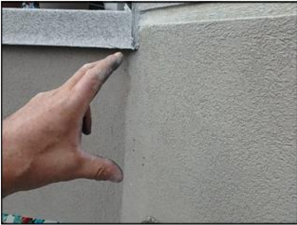
Inconclusive probing results below deck due to OSB substrate cut out to accommodate steel bracket installation; recommend random intrusive evaluation upon system remediation to determine framing condition; typical
