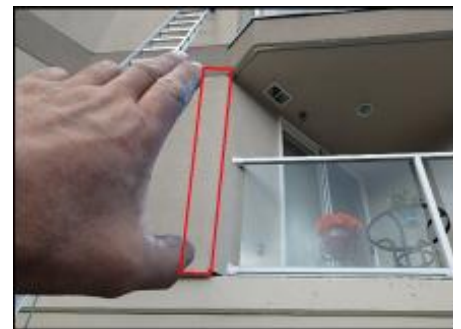
Approximate area of soft substrate needs to be removed and replaced (H5)
