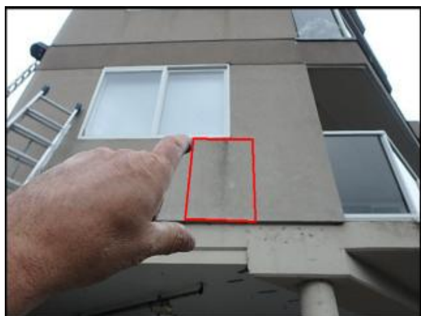
Approximate area of soft substrate needs to be removed and replaced (I6-17)
