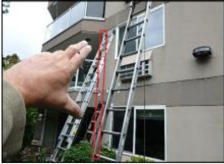
Approximate area of soft substrate needs to be removed and replaced (C5-C7)
