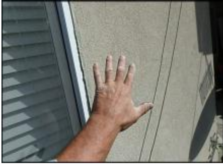
Area of insufficiently attached EIFS needs fasteners installed prior to base coat, mesh and finish coat application; typical
