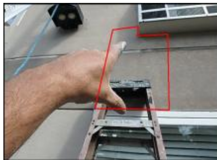
Approximate area of soft substrate needs to be removed and replaced (E5-F6)
