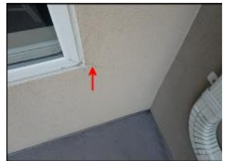
Crack needs to be gouged and slivered with EPS prior to base coat, mesh and finish coat application; typical
