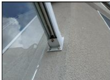
Railing fasteners need to be sealed; typical
