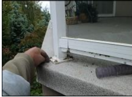
Railing fasteners need to be sealed; typical
