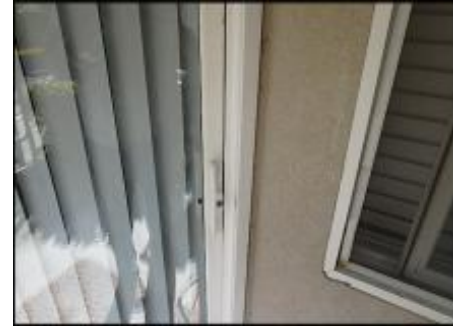
7/8" EIFS needs to be removed at interior deck door head and jambs prior to base coat and mesh application to accommodate 3/4" silicone sealant joint application; typical
