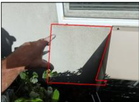
Approximate area of soft substrate needs to be removed and replaced (I6)
