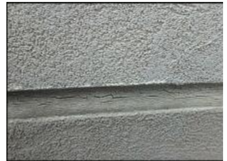
Sealant at floor line expansion joint needs to be removed and EIFS removed at base of joint prior to base coat, mesh and silicone sealant joint application; typical
