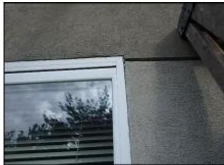
7/8" EIFS needs to be removed at window perimeter prior to base coat and mesh application to accommodate 3/4" silicone sealant joint application; typical
