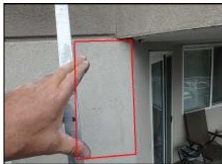
Approximate area of soft substrate needs to be removed and replaced (E4)
