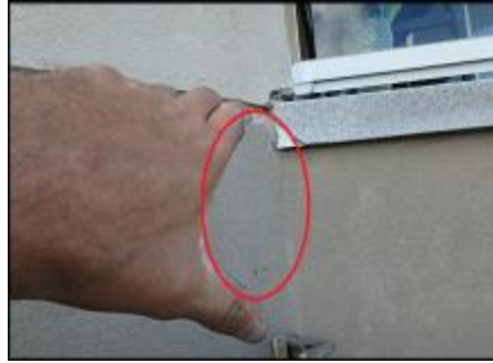
Inconclusive probing results below deck due to OSB substrate cut out to accommodate steel bracket installation; recommend random intrusive evaluation upon system remediation to determine framing condition; typical
