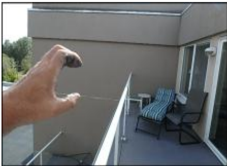
EIFS installed over concrete wall (H2-H6)
