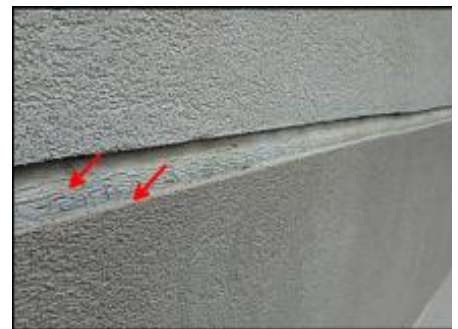
Sealant at floor line expansion joint needs to be removed and EIFS removed at base of joint prior to base coat, mesh and silicone sealant joint application; typical
