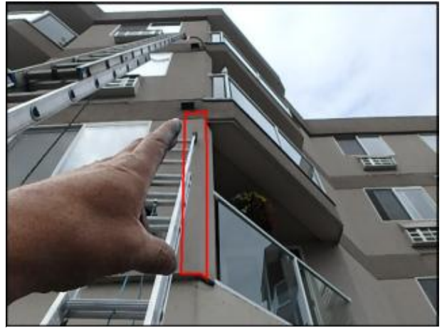
Approximate area of soft substrate needs to be removed and replaced (H4-H6)
