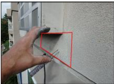
Approximate area of soft substrate needs to be removed and replaced (F3)
