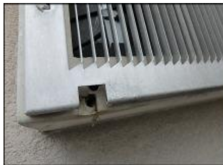
PTAC needs factory drip tubes installed to divert water away from system; typical
