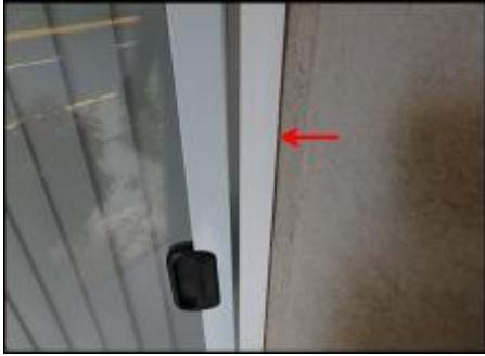
7/8" EIFS needs to be removed at interior deck door head and jambs prior to base coat and mesh application to accommodate 3/4" silicone sealant joint application; typical
