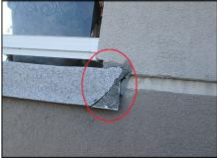
Recommend replacement of deck membrane due to installation defects and failure observed; deck termination needs end dam flashing installed; typical
