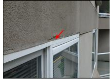
7/8" EIFS needs to be removed at window perimeter prior to base coat and mesh application to accommodate 3/4" silicone sealant joint application; typical
