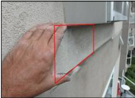
Approximate area of soft substrate needs to be removed and replaced (F3-G3)
