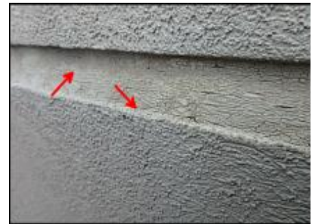
Sealant at floor line expansion joint needs to be removed and EIFS removed at base of joint prior to base coat, mesh and silicone sealant joint application; typical
