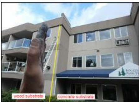
Wood to concrete substrate needs expansion joint installation (H1-H8)
