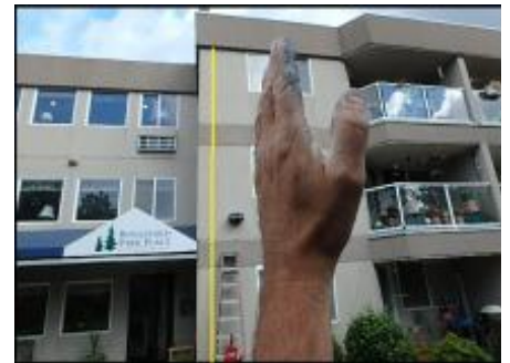
Concrete substrate to wood substrate needs expansion joint installation (D1-E8)
