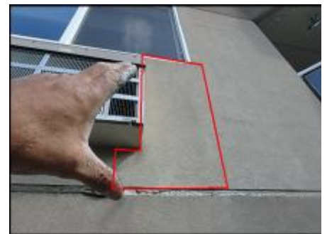
Approximate area of soft substrate needs to be removed and replaced (F5)
