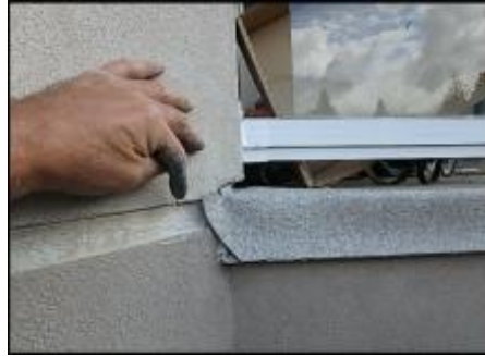
Recommend replacement of deck membrane due to installation defects and failure observed; deck termination needs end dam flashing installation; typical
