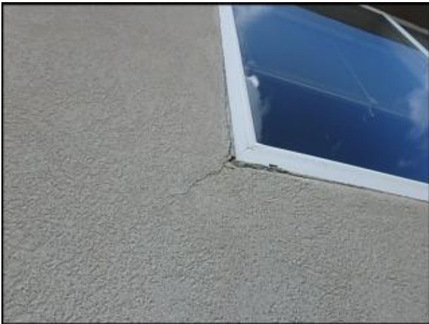
Area of insufficiently attached EIFS needs fasteners installed prior to base coat, mesh and finish coat application over entire system; typical
