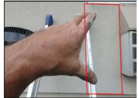
Approximate area of soft substrate needs to be removed and replaced (G5)
