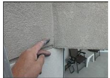
Crack needs to be gouged and slivered with EPS prior to base coat, mesh and finish coat application; typical
