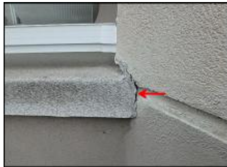
Deck termination needs end dam flashing installation; typical
