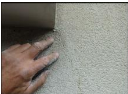
Crack needs to be gouged and slivered with EPS prior to base coat, mesh and finish coat application; typical
