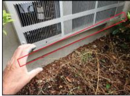
Approximate area of soft substrate needs to be removed and replaced (A7)
