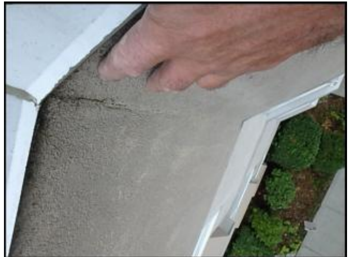
Larger crack at fascia needs to be gouged and slivered with EPS prior to panzer mesh corner installation due to lack of backing at framing members; typical
