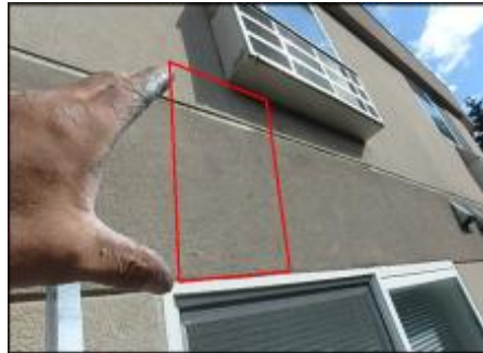
Approximate area of soft substrate needs to be removed and replaced (I4)
