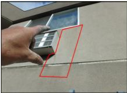
Approximate area of soft substrate needs to be removed and replaced (D3-D4)
