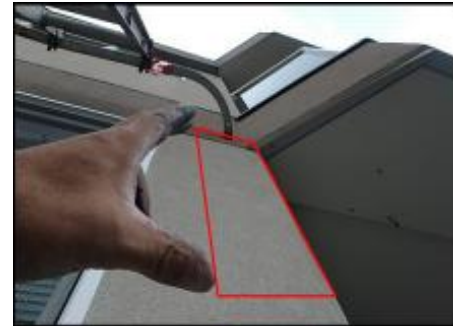
Approximate area of soft substrate needs to be removed and replaced (D4-C4)
