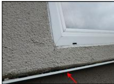
Floor line flashing not adequately extended over EIFS needs sealant joint application (B5-G5)
