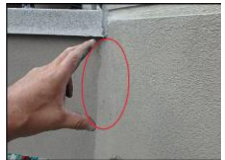
Inconclusive probing results below deck due to OSB substrate cut out to accommodate steel bracket installation; recommend random intrusive evaluation upon system remediation to determine framing condition; typical
