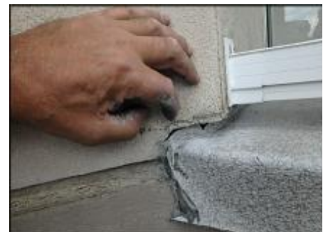
Recommend replacement of deck membrane due to installation defects and failure observed; typical
