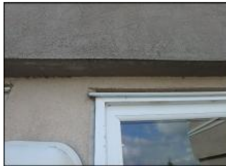
Head flashings installed at window heads; 3/4" sealant joint installed at window jambs and sills (H3-J3)
