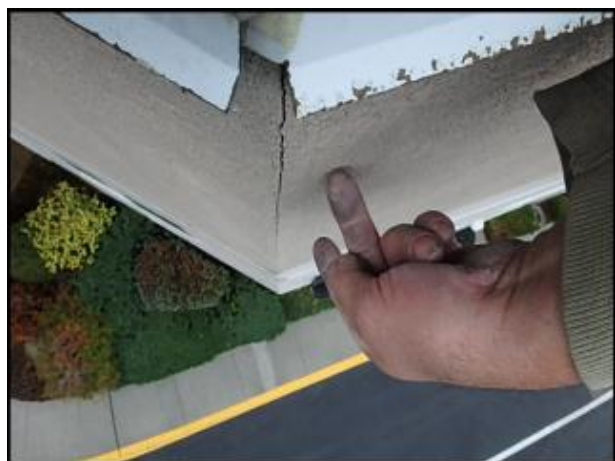
Larger crack at fascia needs to be gouged and slivered with EPS prior to panzer mesh corner installation due to lack of backing at framing members; typical
