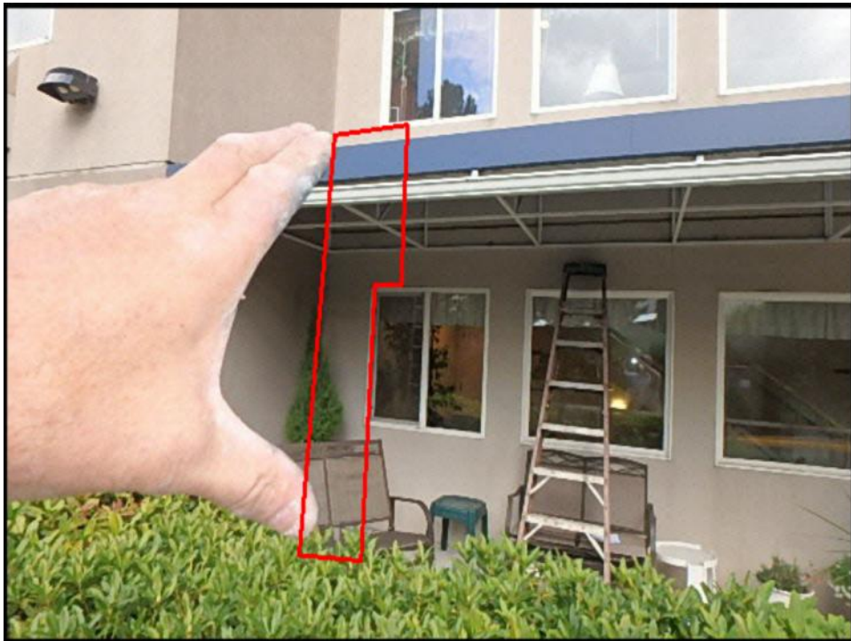
Approximate area of soft substrate needs to be removed and replaced (I5-I8)
