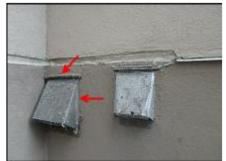
7/8" EIFS needs to be removed at vents prior to base coat and mesh application to accommodate 3/4" silicone sealant joint application; recommend replacing vents upon system remediation; typical
