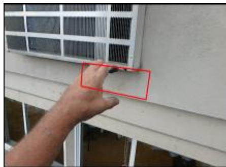
Approximate area of soft substrate needs to be removed and replaced (H5)
