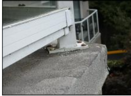
Recommend replacement of deck membrane due to installation defects and aging; typical
