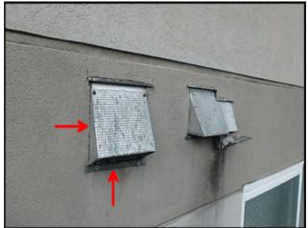
7/8" EIFS needs to be removed at vents prior to base coat and mesh application to accommodate 3/4" silicone sealant joint application; recommend replacing vents upon system remediation; typical
