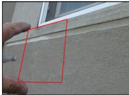
Approximate area of soft substrate needs to be removed and replaced (G5)
