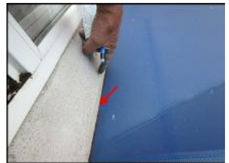
Awning to EIFS needs sealant joint application (I5-J5)
