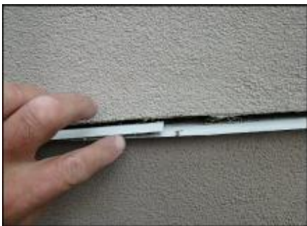
Floor line flashing lap needs to be sealed; typical
