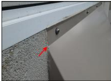
PTAC shroud terminations need remediation to accommodate 1/2" sealant joint application; typical
