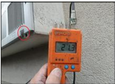
PTAC needs factory drip tubes installed to divert water away from system; typical
