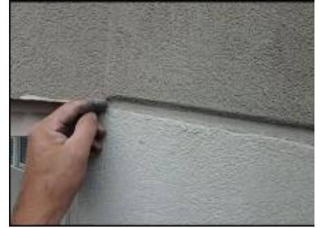
7/8" Sprint board application does not allow for minimum 3/4" foam at base of v-groove; hairline cracks observed; detail needs bond breaker tape and silicone sealant joint application; typical
