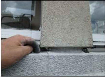
Recommend replacement of deck membrane due to installation defects and failure observed; typical
