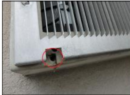
PTAC needs factory drip tubes installed to divert water away from system; typical
