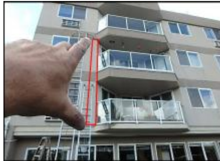
Approximate area of soft substrate needs to be removed and replaced (H5)
