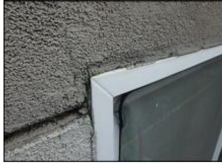
7/8" EIFS needs to be removed at window perimeter prior to base coat and mesh application to accommodate 3/4" silicone sealant joint application; typical
