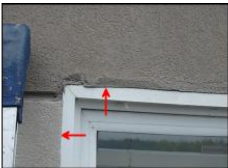
7/8" EIFS needs to be removed at window perimeter prior to base coat and mesh application to accommodate 3/4" silicone sealant joint application; typical
