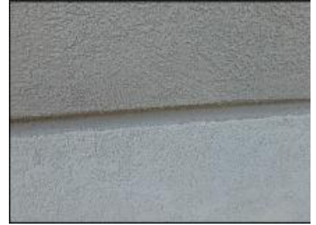
7/8" Sprint board application does not allow for minimum 3/4" foam at base of v-groove; hairline cracks observed; detail needs bond breaker tape and silicone sealant joint application; typical
