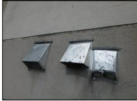
7/8" EIFS needs to be removed at vents prior to base coat and mesh application to accommodate 3/4" silicone sealant joint application; recommend replacing vents upon system remediation; typical
