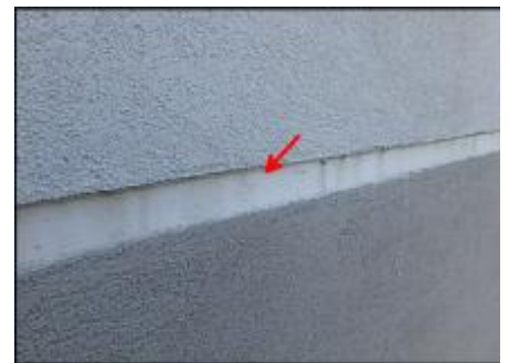
Sealant at floor line expansion joint needs to be removed and EIFS removed at base of joint prior to base coat, mesh and silicone sealant joint application; typical
