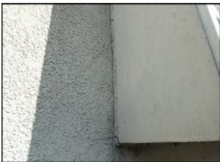
7/8" EIFS needs to be removed at PTAC perimeter prior to base coat and mesh application to accommodate 3/4" silicone sealant joint application; typical
