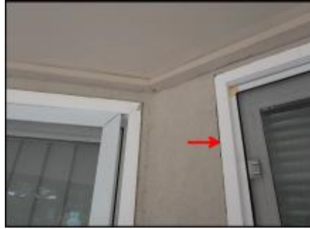
7/8" EIFS needs to be removed at interior deck window perimeter prior to base coat and mesh application to accommodate 3/4" silicone sealant joint application; typical
