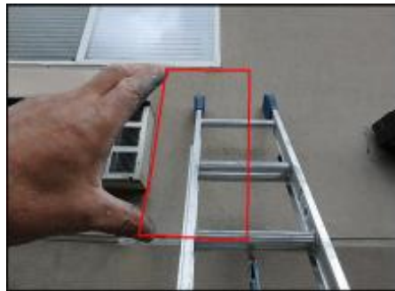
Approximate area of soft substrate needs to be removed and replaced (B6)
