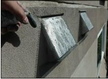
7/8" EIFS needs to be removed at vents prior to base coat and mesh application to accommodate 3/4" silicone sealant joint application; recommend replacing vents upon system remediation; typical
