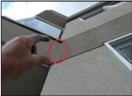
Inconclusive probing results below deck due to OSB substrate cut out to accommodate steel bracket installation; recommend random intrusive evaluation upon system remediation to determine framing condition; typical
