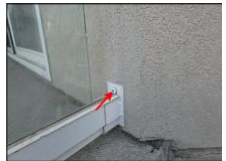
Railing fasteners need to be sealed; typical
