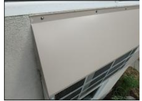
PTAC shroud terminations need remediation to accommodate 1/2" sealant joint application; typical
