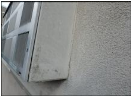
7/8" EIFS needs to be removed at PTAC perimeter prior to base coat and mesh application to accommodate 3/4" silicone sealant joint application; typical
