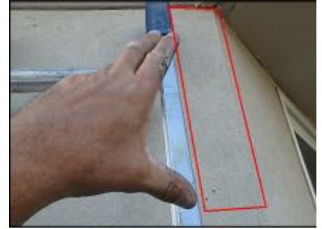
Approximate area of soft substrate needs to be removed and replaced (B4)
