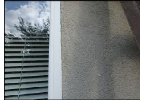
Area of insufficiently attached EIFS needs fasteners installed prior to base coat, mesh and finish coat application; typical
