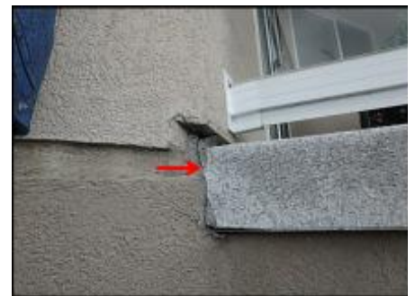
Deck termination needs end dam flashing installation; typical
