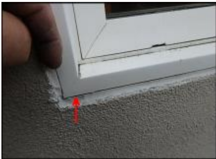
Sealant failure observed at window jambs and sill (C4-C7)
