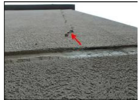
Movement crack observed at wood substrate to concrete substrate (H1-H3)
