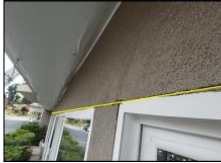
Window heads need expansion joint installation (D6-H6)
