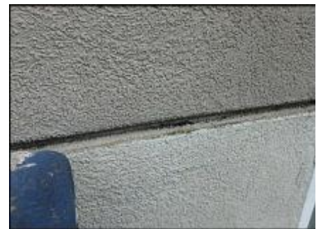
7/8" Sprint board application does not allow for minimum 3/4" foam at base of v-groove; hairline cracks observed; detail needs bond breaker tape and silicone sealant joint application; typical
