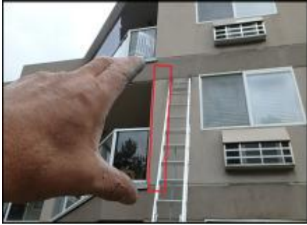
Approximate area of soft substrate needs to be removed and replaced (A5-A6)
