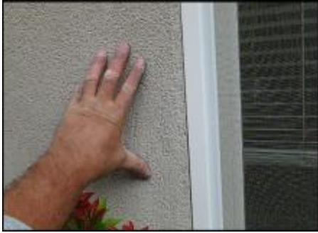
Area of insufficiently attached EIFS needs fasteners installed prior to base coat, mesh and finish coat application; typical
