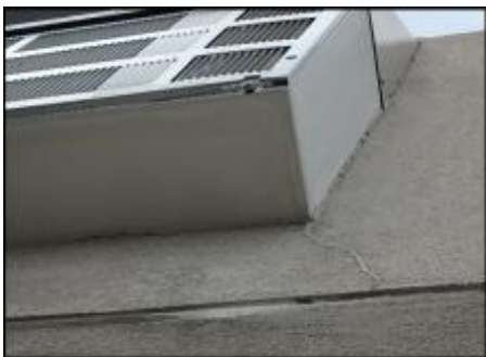
Cracks need to be gouged and slivered with EPS prior to base coat, mesh and finish coat application; typical
