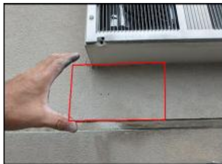
Approximate area of soft substrate needs to be removed and replaced (A5-B5)
