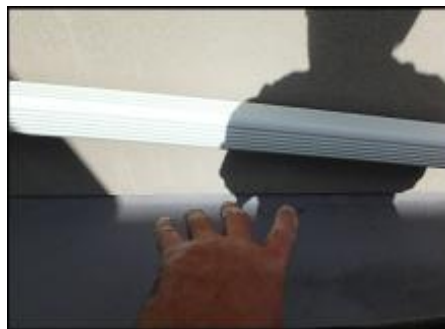
Hairline cracks will be remediated with application of base coat, mesh and finish coat application over entire system; typical
