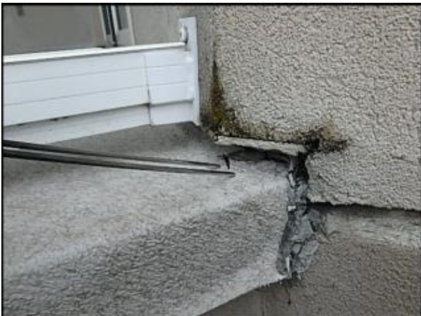
Recommend replacement of deck membrane due to installation defects and failure observed; typical
