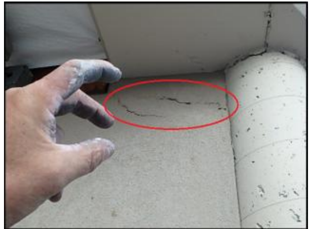
Compression damage needs to be gouged and slivered with EPS prior to base coat, mesh and finish coat application (J6)
