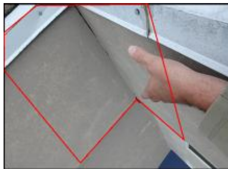
Approximate area of soft substrate needs to be removed and replaced (H1-I2)
