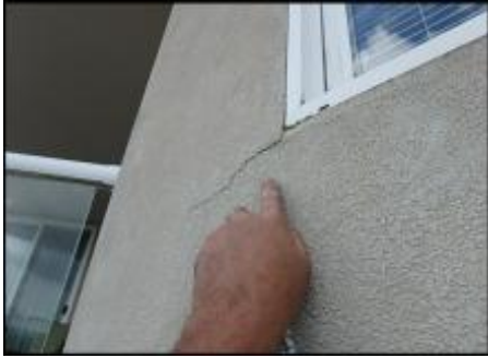
Crack needs to be gouged and slivered with EPS prior to base coat, mesh and finish coat application; typical
