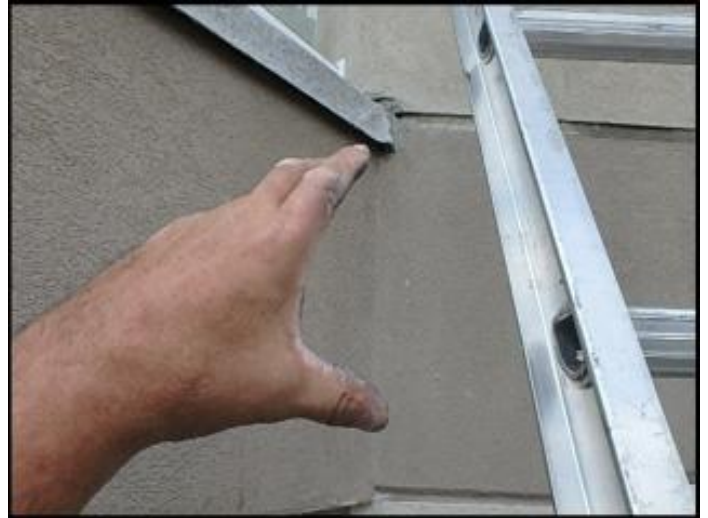
Inconclusive probing results below deck due to OSB substrate cut out to accommodate steel bracket installation; recommend random intrusive evaluation upon system remediation to determine framing condition; typical
