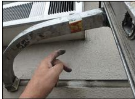
Crack needs to be gouged and slivered with EPS prior to base coat, mesh and finish coat application; typical
