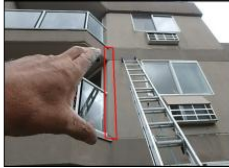
Approximate area of soft substrate needs to be removed and replaced (E4-E5)
