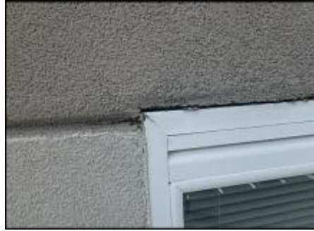
7/8" EIFS needs to be removed at window perimeter prior to base coat and mesh application to accommodate 3/4" silicone sealant joint application; typical
