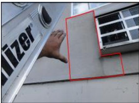
Approximate area of soft substrate needs to be removed and replaced (E6-F6)
