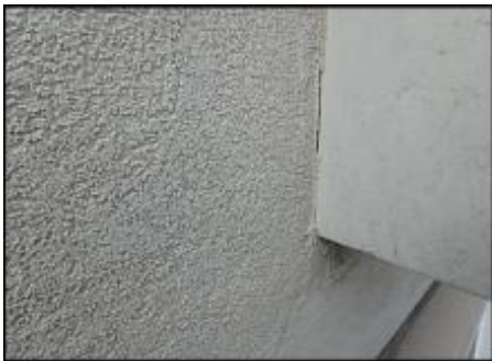
7/8" EIFS needs to be removed at PTAC perimeter prior to base coat and mesh application to accommodate 3/4" silicone sealant joint application; typical
