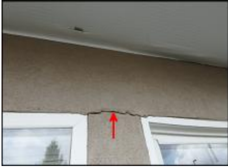
Area of compression damage needs expansion joint installation (D6-H6)
