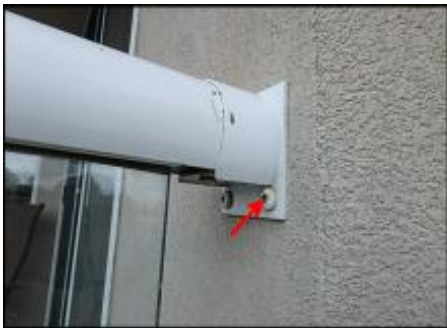
Railing fasteners need to be sealed; typical
