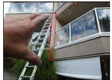
Approximate area of soft substrate needs to be removed and replaced (B4-B5)
