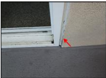
Sealant joint failure at door jamb needs to be removed and replaced (H3)
