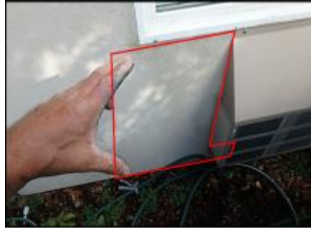
Approximate area of soft substrate needs to be removed and replaced (C6)
