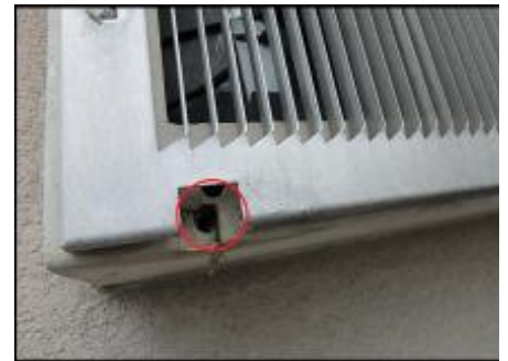
PTAC needs factory drip tubes installed to divert water away from system; typical
