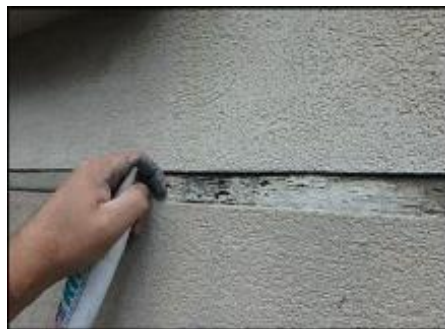
Sealant at floor line expansion joint needs to be removed and EIFS removed at base of joint prior to base coat, mesh and silicone sealant joint application; typical
