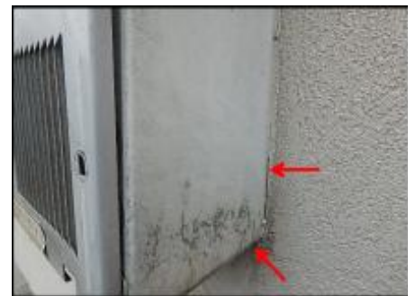
7/8" EIFS needs to be removed at PTAC perimeter prior to base coat and mesh application to accommodate 3/4" silicone sealant joint application; typical
