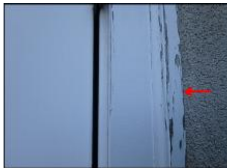
7/8" EIFS needs to be removed at door jambs prior to base coat and mesh application to accommodate 3/4" silicone sealant joint application; typical (H7)
