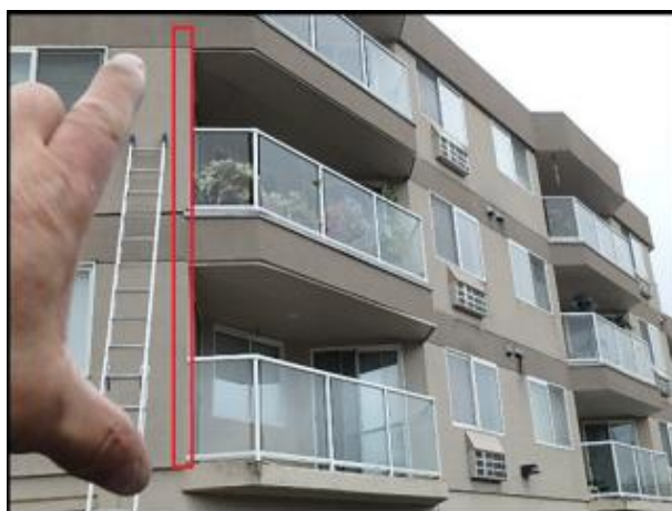
Approximate area of soft substrate needs to be removed and replaced (I3-J7)
