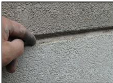
7/8" Sprint board application does not allow for minimum 3/4" foam at base of v-groove; hairline cracks observed; detail needs bond breaker tape and silicone sealant joint application; typical
