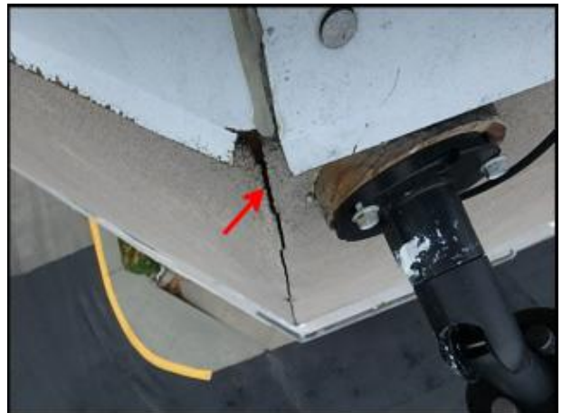
Crack needs to be gouged and slivered with EPS prior to panzer corner mesh application; typical
