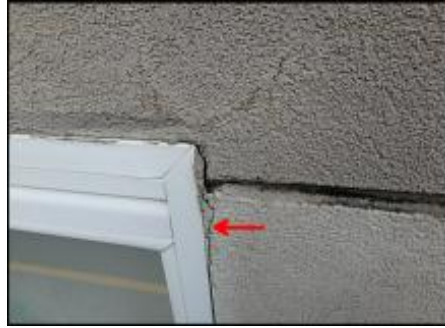
7/8" EIFS needs to be removed at window perimeter prior to base coat and mesh application to accommodate 3/4" silicone sealant joint application; typical
