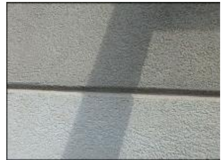
7/8" Sprint board application does not allow for minimum 3/4" foam at base of v-groove; hairline cracks observed; detail needs bond breaker tape and silicone sealant joint application; typical
