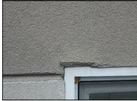
7/8" EIFS needs to be removed at window perimeter prior to base coat and mesh application to accommodate 3/4" silicone sealant joint application; typical
