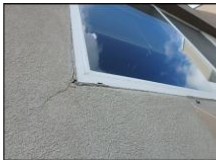
Area of insufficiently attached EIFS needs fasteners installed prior to base coat, mesh and finish coat application; typical
