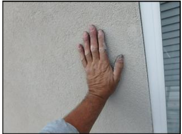
Area of insufficiently attached EIFS needs fasteners installed prior to base coat, mesh and finish coat application; typical
