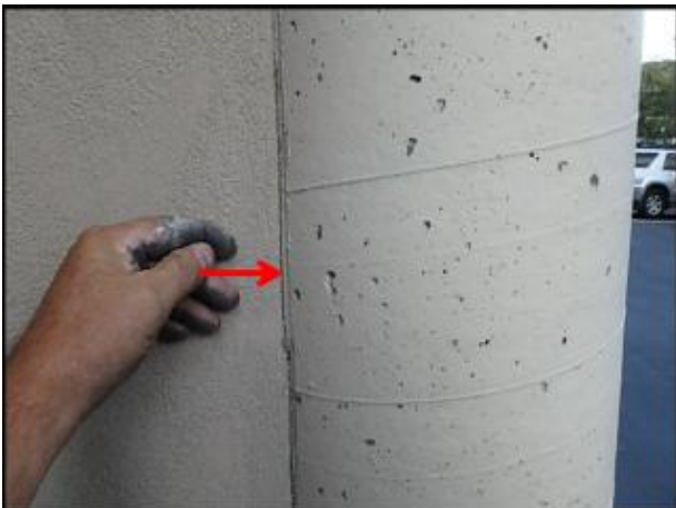
7/8" EIFS needs to be removed at column prior to base coat and mesh application to accommodate 3/4" silicone sealant joint application (J6-J7)
