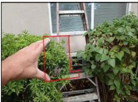
Approximate area of soft substrate needs to be removed and replaced (B7)
