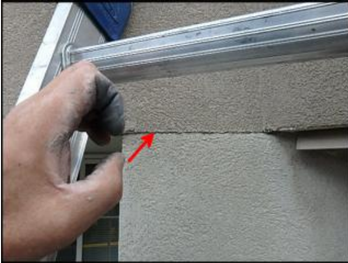
Crack needs to be gouged and slivered with EPS prior to base coat, mesh and finish coat application; typical
