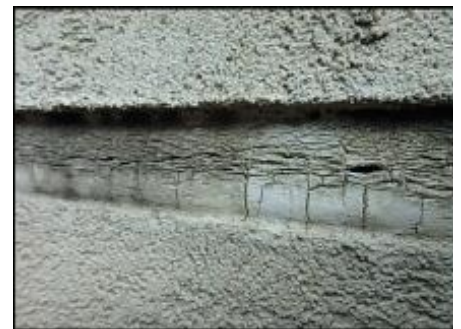
Sealant at floor line expansion joint needs to be removed and EIFS removed at base of joint prior to base coat, mesh and silicone sealant joint application; typical
