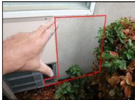
Approximate area of soft substrate needs to be removed and replaced (G8)
