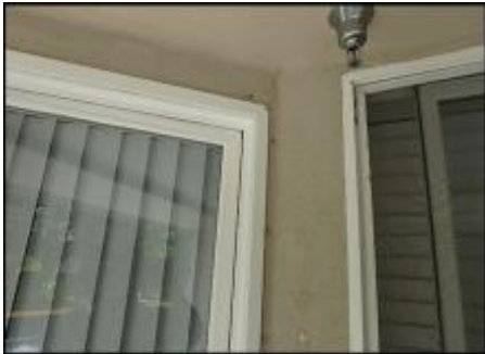
7/8" EIFS needs to be removed at interior deck window perimeter prior to base coat and mesh application to accommodate 3/4" silicone sealant joint application; typical
