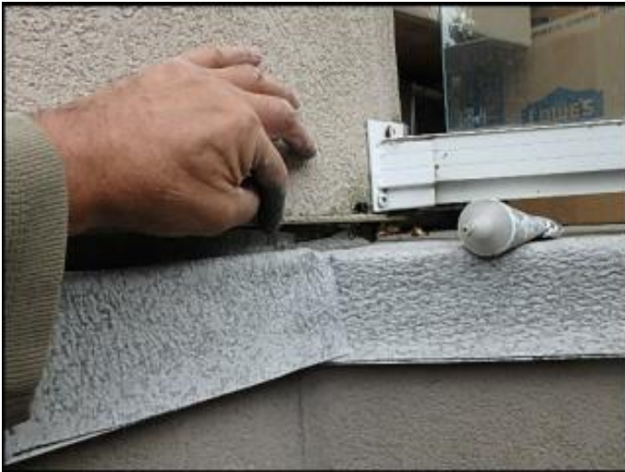
Recommend replacement of deck membrane due to installation defects and failure observed; typical
