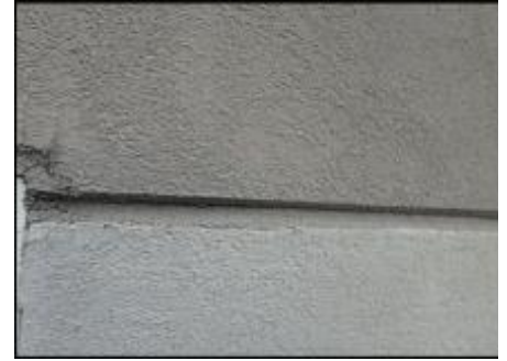
7/8" Sprint board application does not allow for minimum 3/4" foam at base of v-groove; hairline cracks observed; detail needs bond breaker tape and silicone sealant joint application; typical
