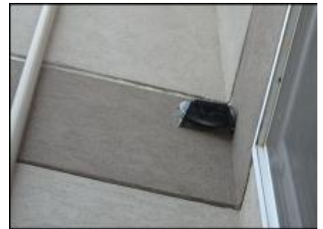
7/8" EIFS needs to be removed at vent prior to base coat and mesh application to accommodate 3/4" silicone sealant joint application; recommend replacing vent upon system remediation; typical
