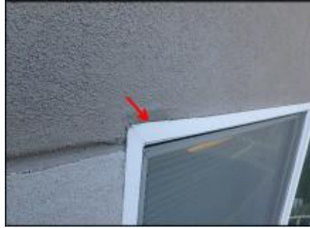
7/8" EIFS needs to be removed at window perimeter prior to base coat and mesh application to accommodate 3/4" silicone sealant joint application; typical
