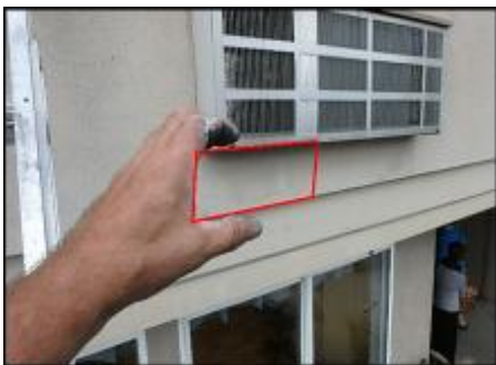
Approximate area of soft substrate needs to be removed and replaced (G5)
