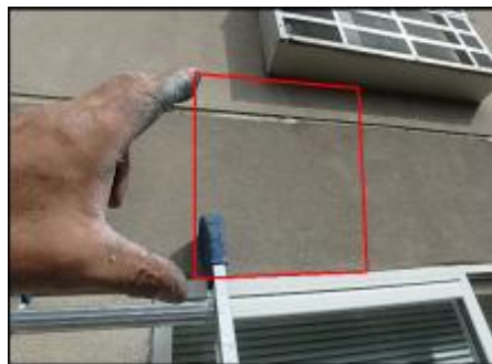
Approximate area of soft substrate needs to be removed and replaced (I4)
