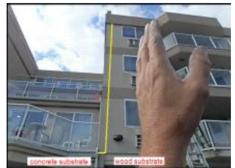
Concrete substrate to wood substrate needs expansion joint installation (C1-C5)
