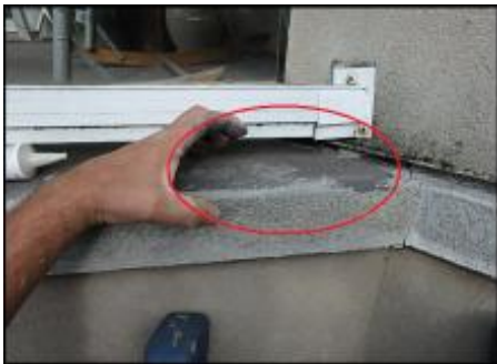
Wood rot detected at deck substrate (B4)
