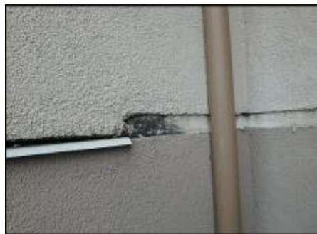
Sealant at floor line expansion joint needs to be removed and EIFS removed at base of joint prior to base coat, mesh and silicone sealant joint application; typical
