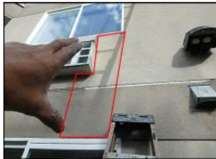
Approximate area of soft substrate needs to be removed and replaced (D5)
