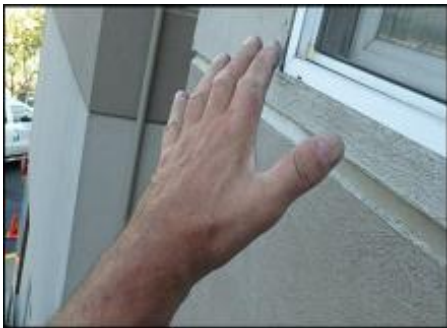
Area of insufficiently attached EIFS needs fasteners installed prior to base coat, mesh and finish coat application; typical
