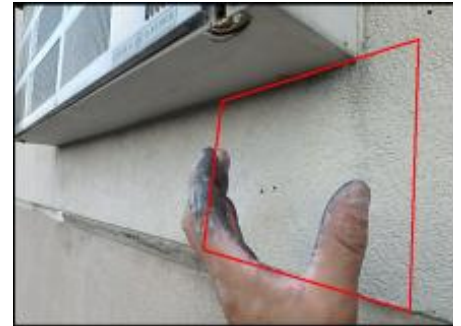
Approximate area of soft substrate needs to be removed and replaced (F5)
