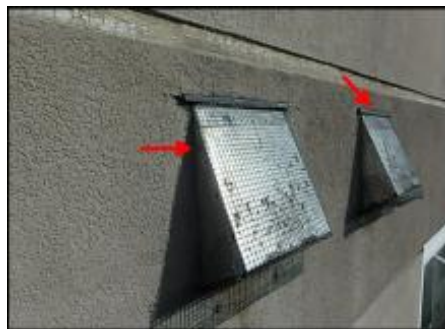
7/8" EIFS needs to be removed at vents prior to base coat and mesh application to accommodate 3/4" silicone sealant joint application; recommend replacing vents upon system remediation; typical
