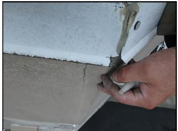
Larger crack at fascia needs to be gouged and slivered with EPS prior to panzer mesh corner installation due to lack of backing at framing members; typical
