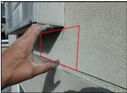
Approximate area of soft substrate needs to be removed and replaced (J4)
