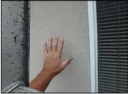
Area of unattached EIFS needs fasteners installed prior to base coat, mesh and finish coat application; typical
