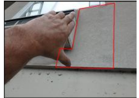
Approximate area of soft substrate needs to be removed and replaced (C5-C6)
