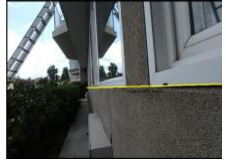
Window sills need expansion joint installation (D6-H6)
