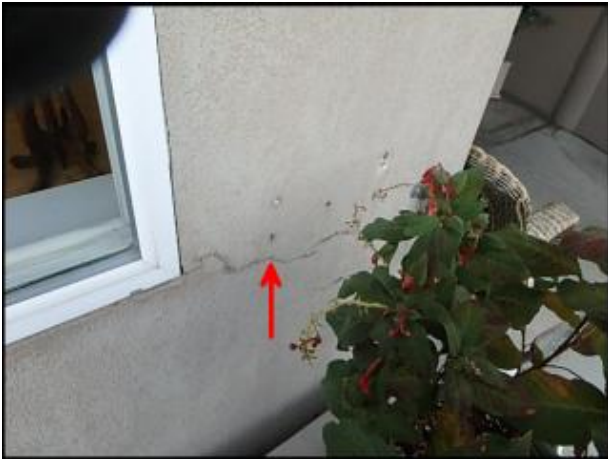
Area of compression damage needs expansion joint installation (H7)
