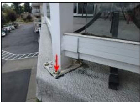
Deck fasteners need to be sealed; typical
