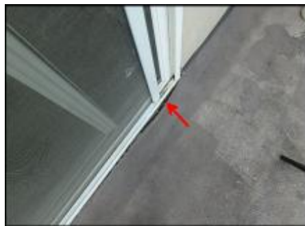
Deck membrane needs to be removed and replaced due to failure observed (H5-J6)
