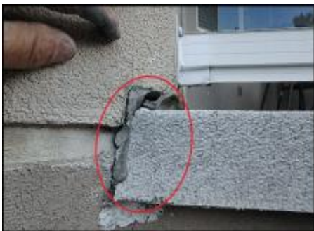
Recommend replacement of deck membrane due to installation defects and failure observed; deck termination needs end dam flashing installation; typical
