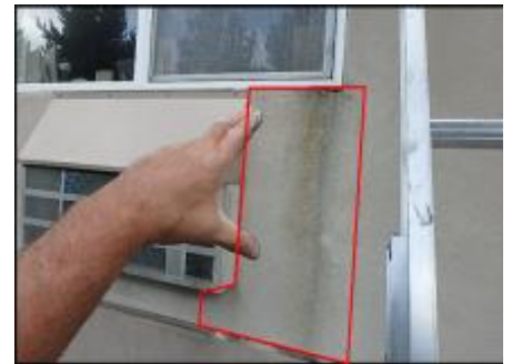
Approximate area of soft substrate needs to be removed and replaced (B6)
