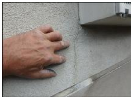
Crack needs to be gouged and slivered with EPS prior to base coat, mesh and finish coat application; typical
