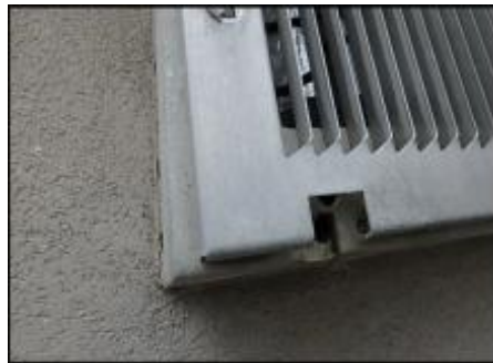
PTAC needs factory drip tubes installed to divert water away from system; typical
