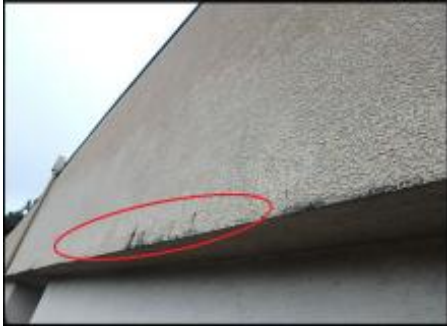
Hairline cracks will be remediated with application of base coat, mesh and finish coat application over entire system; typical
