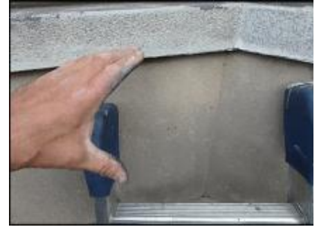
Inconclusive probing results below deck due to OSB substrate cut out to accommodate steel bracket installation; recommend random intrusive evaluation upon system remediation to determine framing condition; typical
