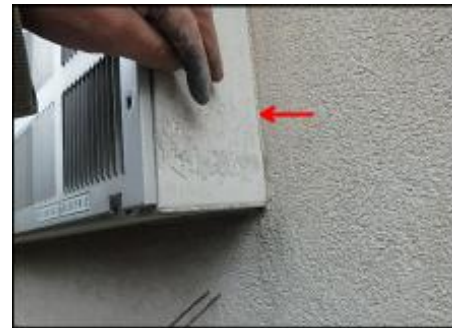
7/8" EIFS needs to be removed at PTAC perimeter prior to base coat and mesh application to accommodate 3/4" silicone sealant joint application; typical
