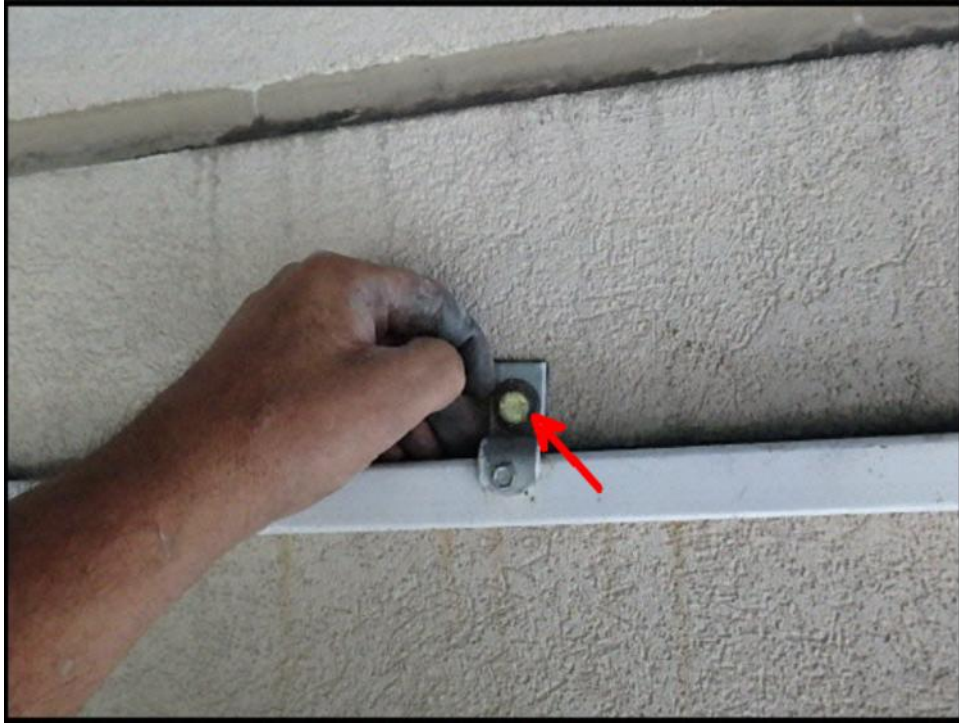
Awning fastener needs sleeve set in bed of sealant application; typical
