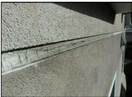
Sealant at floor line expansion joint needs to be removed and EIFS removed at base of joint prior to base coat, mesh and silicone sealant joint application; typical
