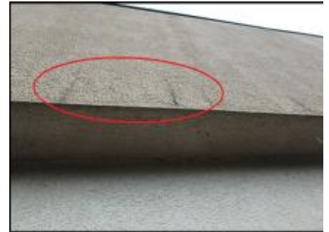
Hairline cracks will be remediated with application of base coat, mesh and finish coat application; typical
