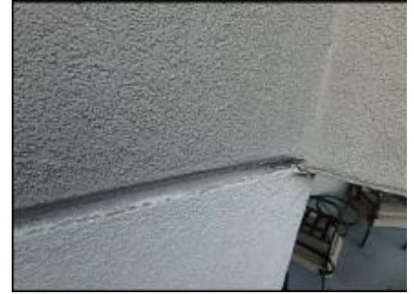
7/8" Sprint board application does not allow for minimum 3/4" foam at base of v-groove; hairline cracks observed; detail needs bond breaker tape and silicone sealant joint application; typical
