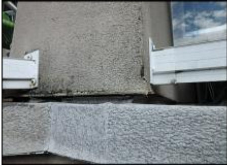
Recommend replacement of deck membrane due to installation details and aging; typical
