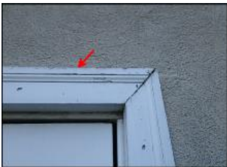
Door head needs drip flashing installation (H7)
