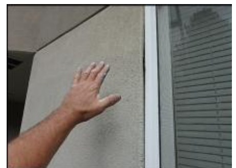
Area of insufficiently attached EIFS needs fasteners installed prior to base coat, mesh and finish coat application; typical
