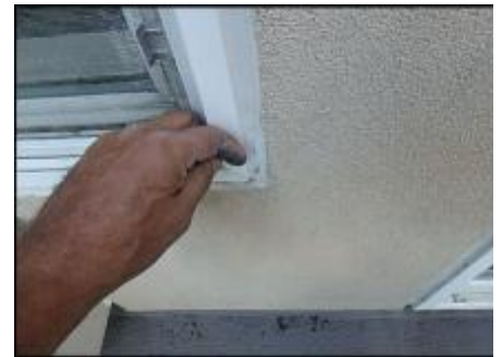
Sealant joint failure at window jamb needs to be removed and replaced (H3)
