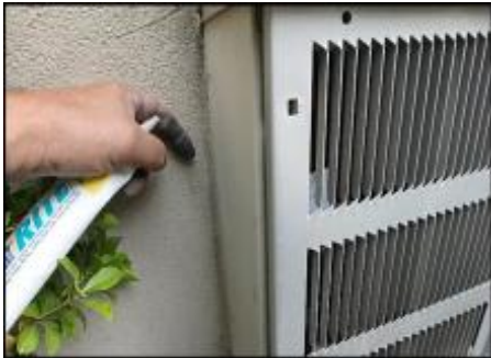
7/8" EIFS needs to be removed at PTAC perimeter prior to base coat and mesh application to accommodate 3/4" silicone sealant joint application; typical
