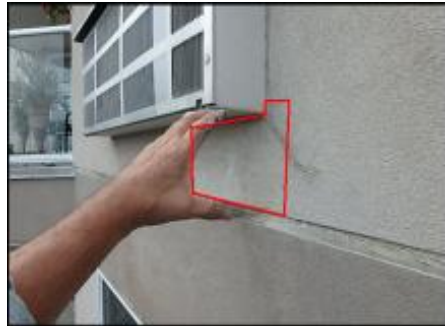
Approximate area of soft substrate needs to be removed and replaced (G3)
