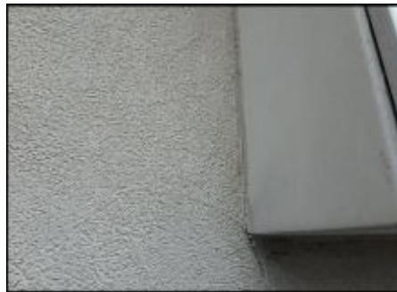
7/8" EIFS needs to be removed at PTAC perimeter prior to base coat and mesh application to accommodate 3/4" silicone sealant joint application; typical
