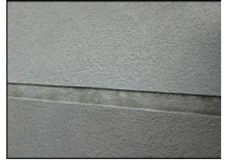
Sealant at floor line expansion joint needs to be removed and EIFS removed at base of joint prior to base coat, mesh and silicone sealant joint application; typical
