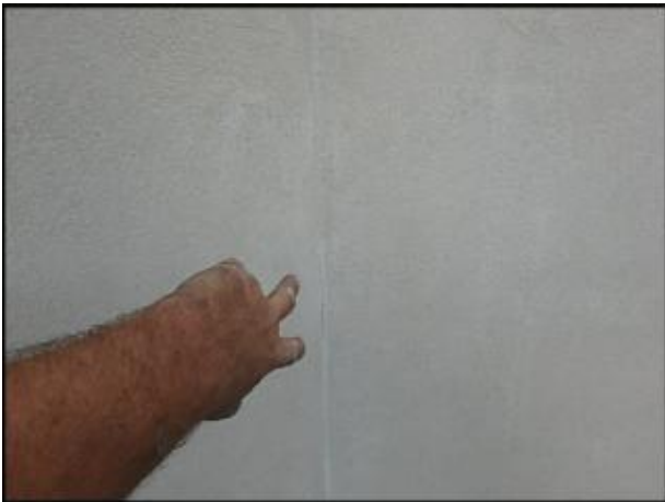
Cracks need to be gouged and slivered with EPS prior to base coat, mesh and finish coat application; typical
