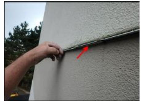
Floor line flashing not adequately extended over EIFS needs sealant joint application (B5-G5)
