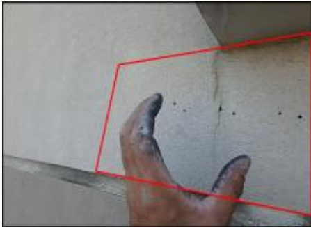
Approximate area of soft substrate needs to be removed and replaced (F3)
