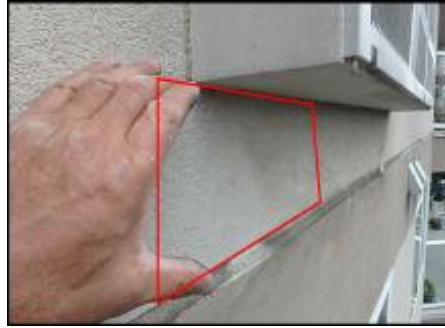
Approximate area of soft substrate needs to be removed and replaced (C4)
