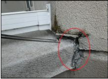
Recommend replacement of deck membrane due to installation defects and failure observed; deck termination needs end dam flashing installation; typical
