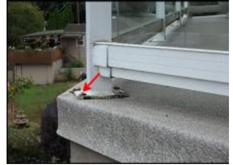
Railing fasteners needs to be sealed; typical
